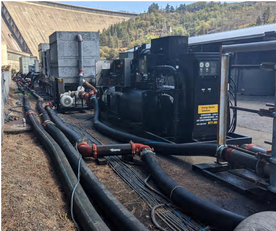
Figure 7 The temporary water chillers and related equipment installed at LSNFH in WY 2121.
