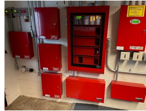
Integrated Fire Alarm Control Panel and Suppression Panels
