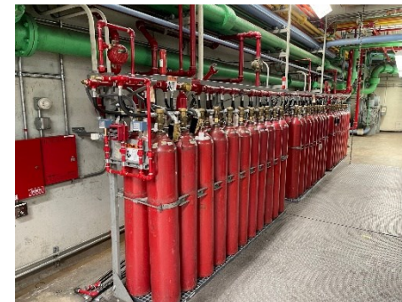
Carbon Dioxide Suppression in generator and transformer housings
