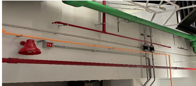
Warning speaker with orange air sampling detection line and fire sprinklers
