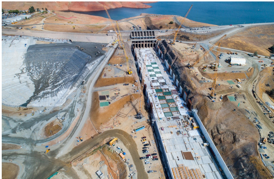
Starting in May 2017, DWR and its construction contractors began repairing and rebuilding Oroville’s main and emergency spillways. As of November 1, 2018, the main spillway was successfully reconstructed, meeting DWR’s public safety construction milestone.
