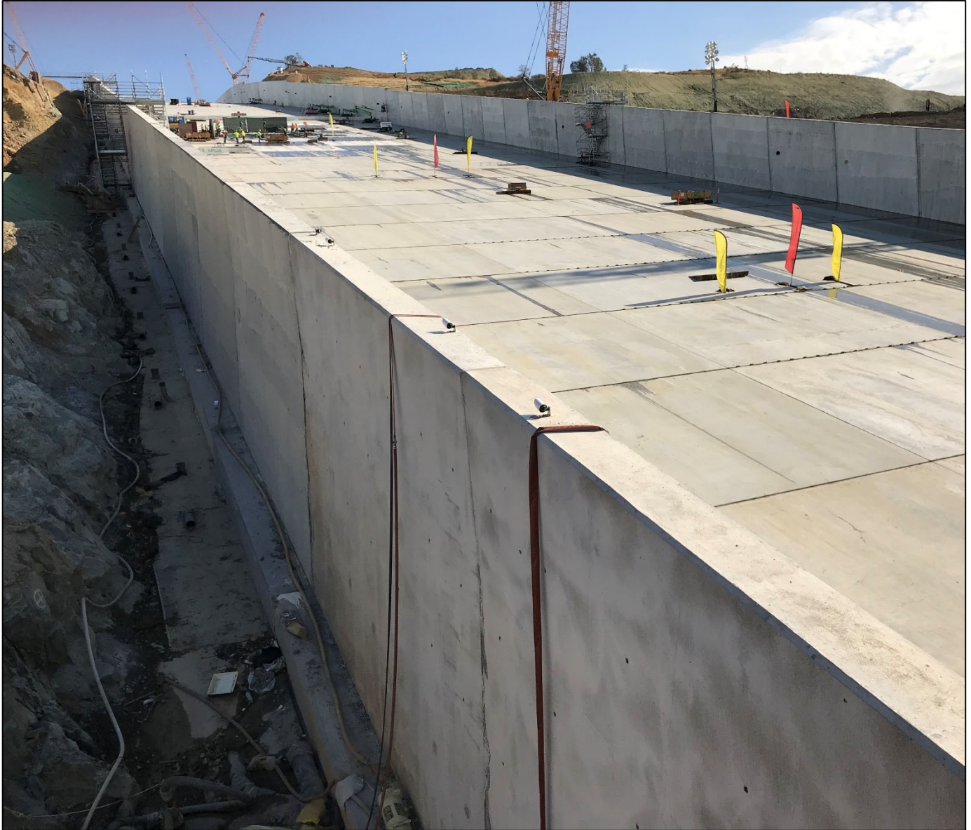
Figure 3. Construction of chute slabs, walls and drains in the middle sections of FCO chute (lower right side).
