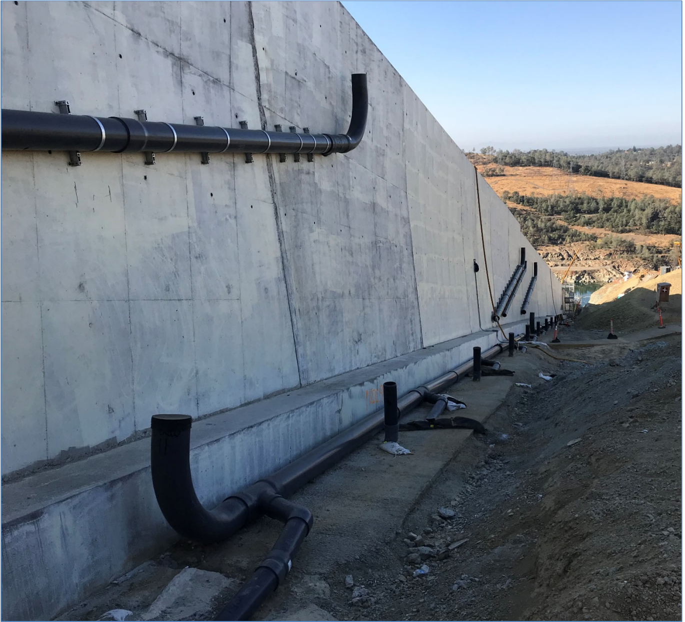
Figure 2. Construction of wall drains in the middle section of FCO chute (middle right side).
