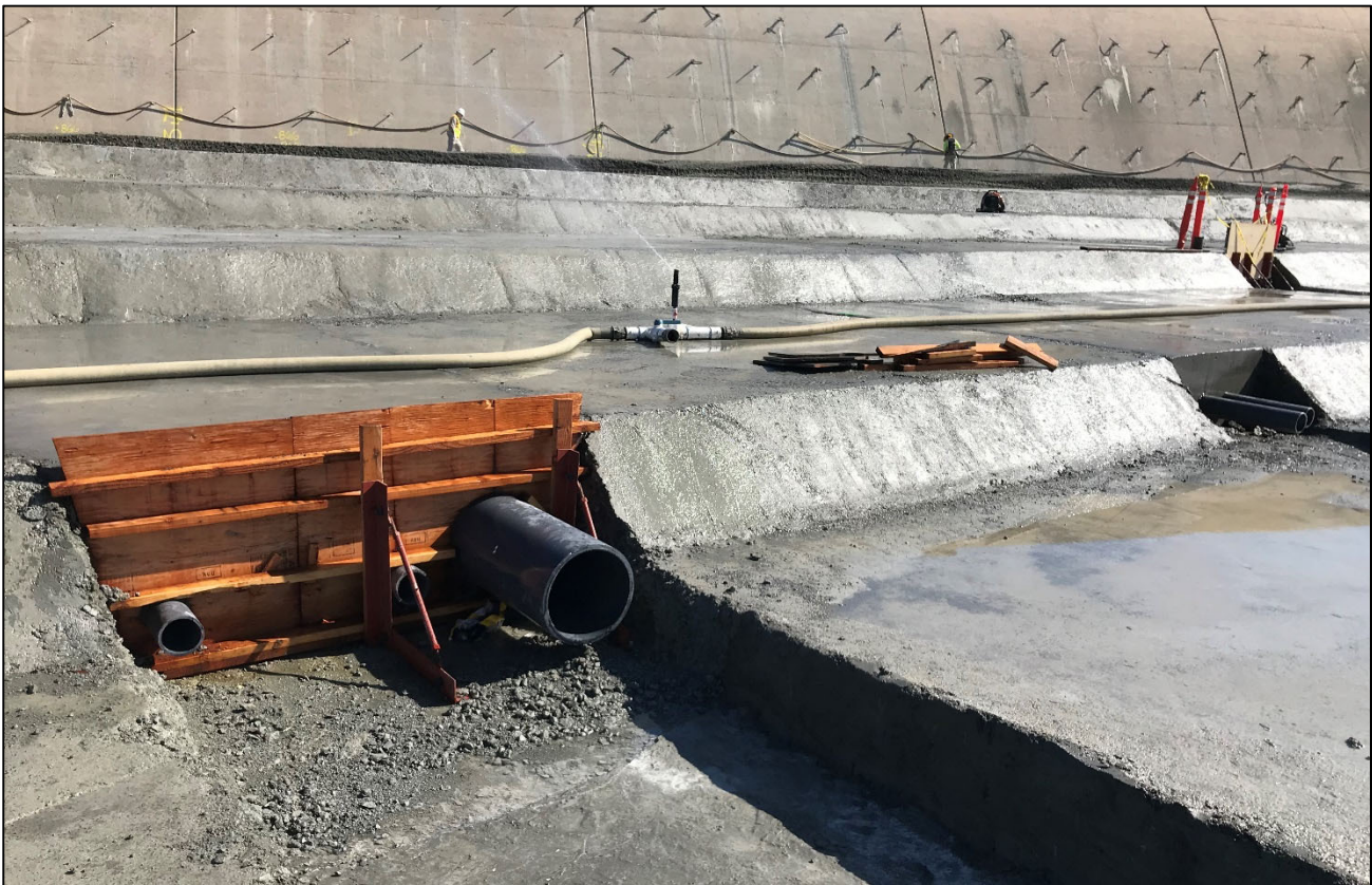
Figure 7. RCC apron, drains, and butress of the ogee monoliths for the Emergency Spillway.
