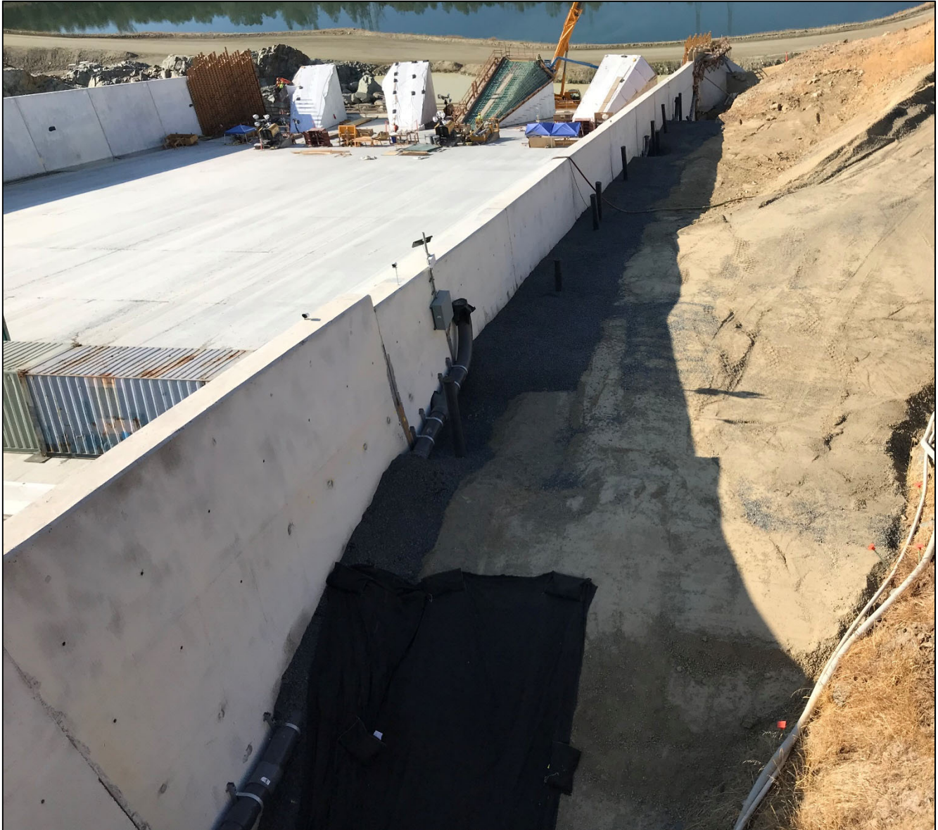
Figure 4. Reconstruction of the terminal structure and backfill along the end section of FCO chute (end of right side).
