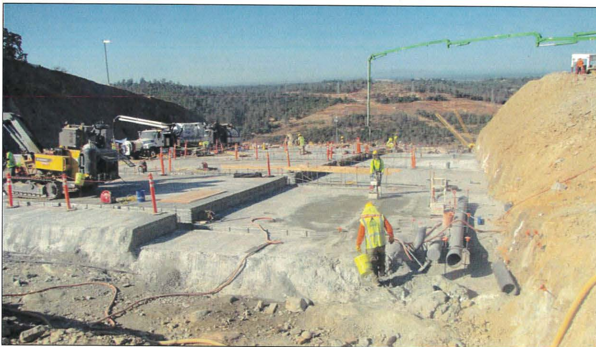
Figure 1. Photographs of typical FCO foundation preparation showing foundation cleanup and Stay-Form (upper photos), and placement of leveling concrete (lower photo).
