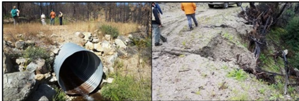
Figure 5 Review team inspecting drainage and erosion issues proximate to harvest site.
