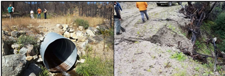
Figure 11: Review team inspecting drainage and erosion issues proximate to harvest site.
