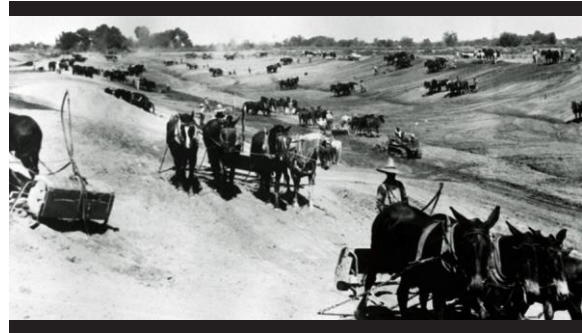
Construction of the All-American Canal with mule teams and Fresno scrapers. Reclamation photo 1935.
