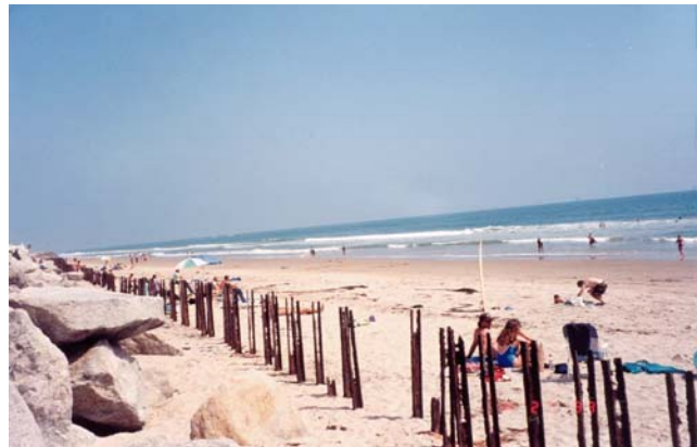
Corroded Railroad Irons, Site 17 Padaro Lane - Santa Clause Lane
