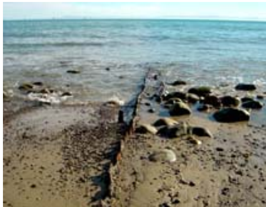
Corroded Sheet Piles, Site 13 Coral Casino -Biltmore Hotel
