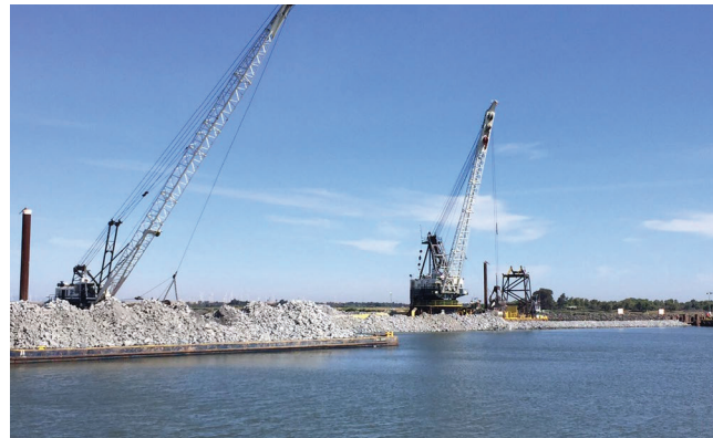
The State installed a salinity drought barrier to stop the encroachment of saline waters into the Sacramento-San Joaquin Delta due to the lack of freshwater flows.
